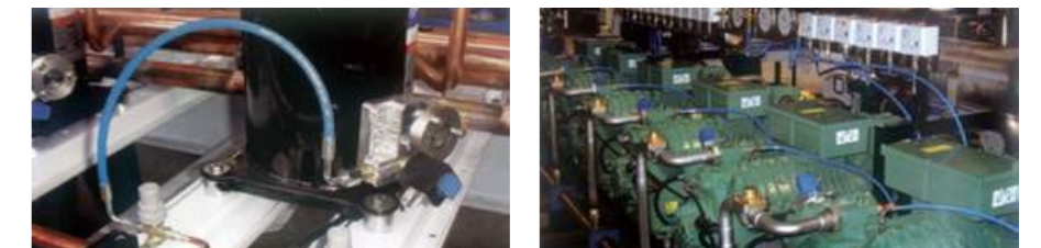
Connection with pressure gauge, control units and oil return pipe.
